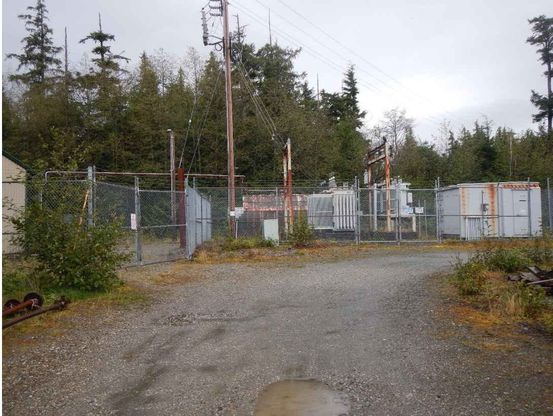
PHOTO 1 – Looking north from the access drive to the middle and eastern portion of the lot. 100920 (89)
