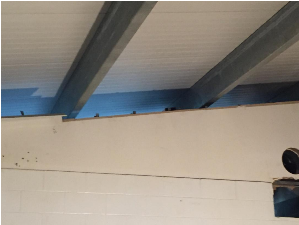
Gap at top of North Women's Locker Room Wall 7-15-16
