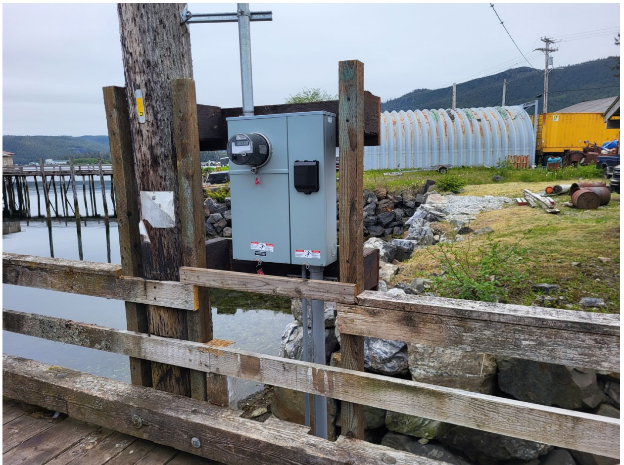
New meter base at head of City Dock
