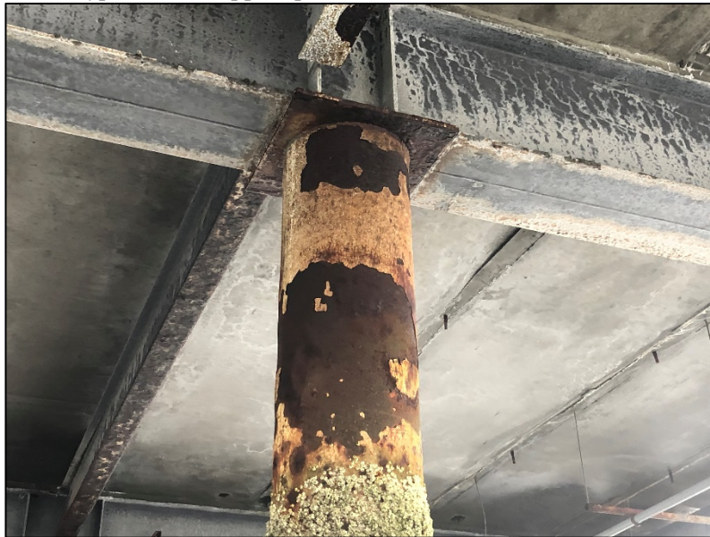
Typical corrosion of steel dock pile in splash zone.
