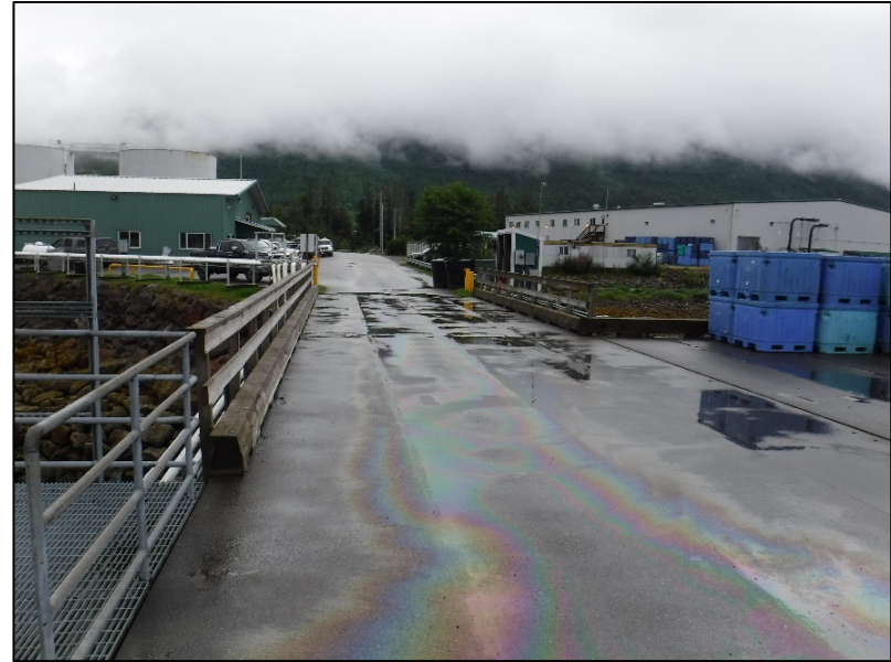
Ponding of water on approach dock deck.
