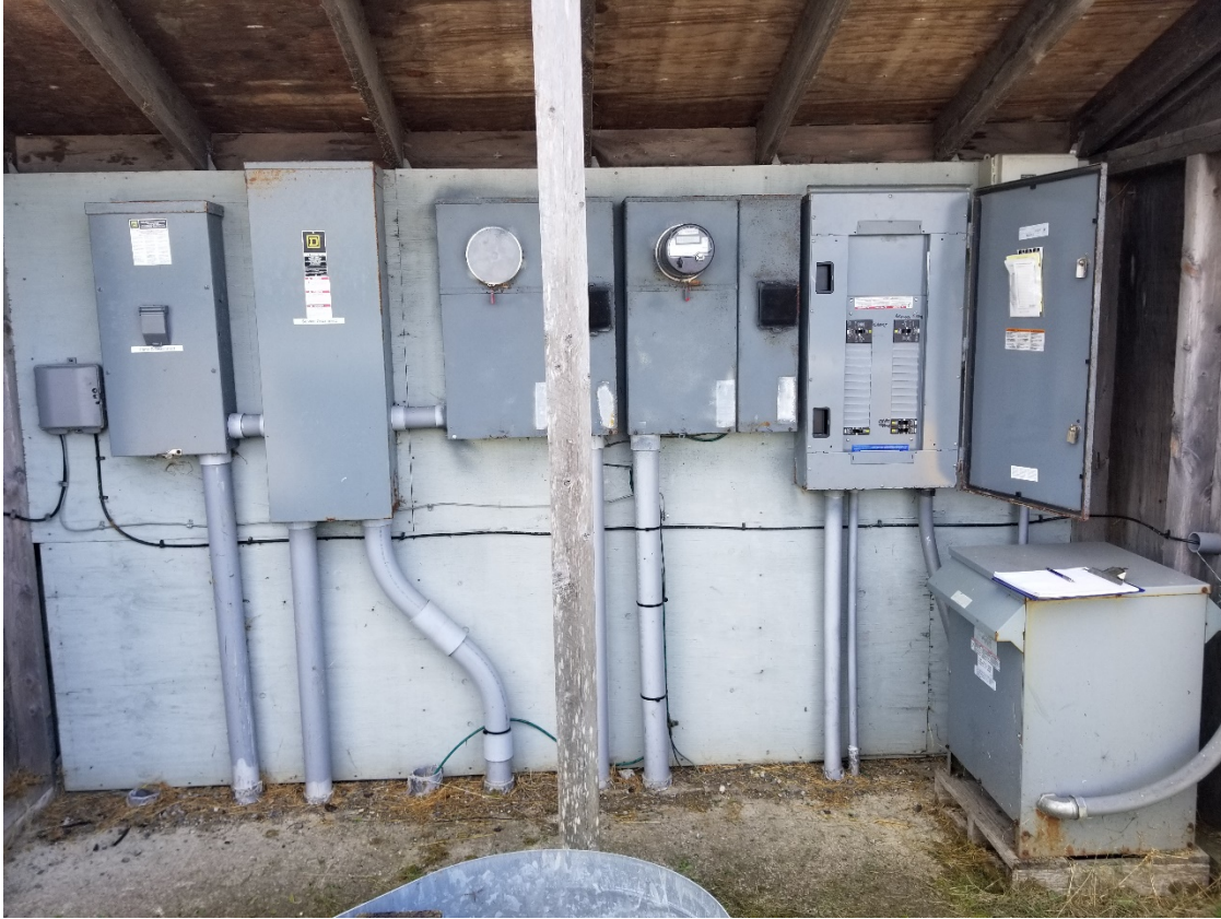
Photo 1: Service Equipment - Three Ice House Main Circuit Breakers on the Left and Dock Circuit Breaker & Distribution Panel on the Right
