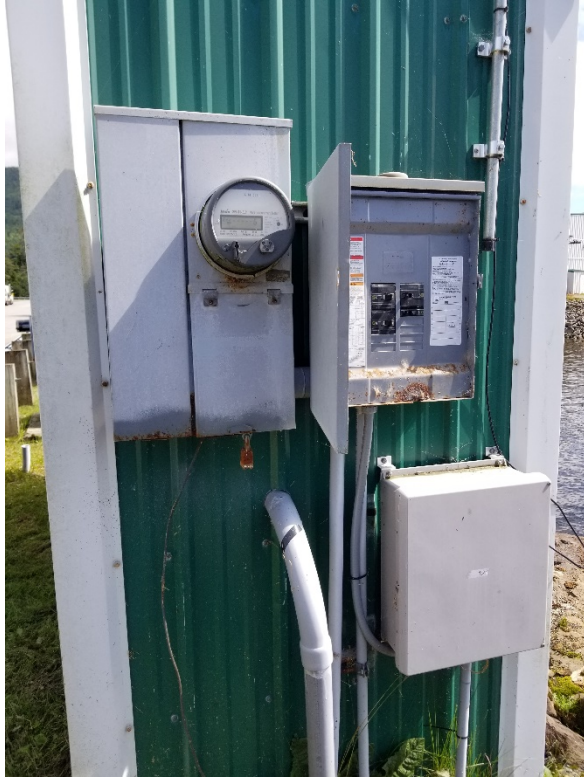
Photo 4: Service Equipment and Panelboard for Refrigerated Containers
