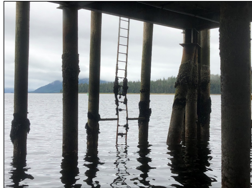
Typical corroded/damaged access ladder.
