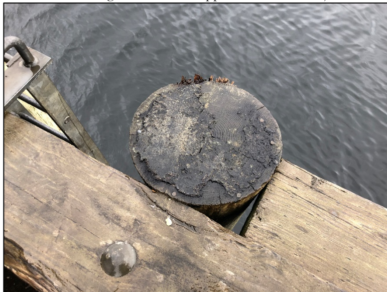
Typical deterioration of fender pile end covering.
