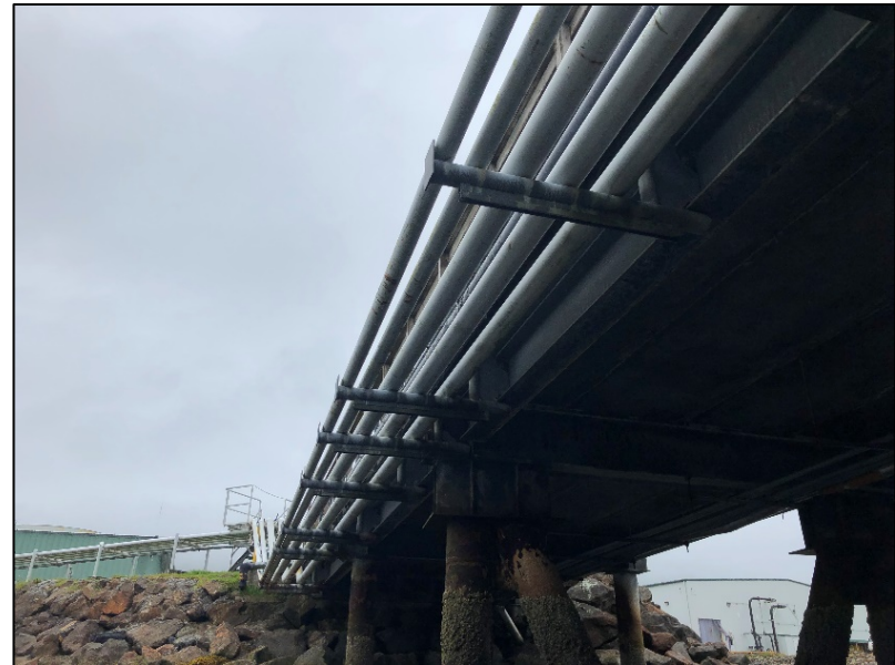
Fuel line routing alongside approach dock (north side).
