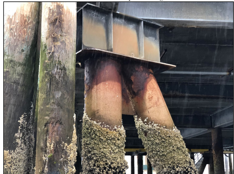
Typical corrosion of steel dock piles in splash zone (above water).
