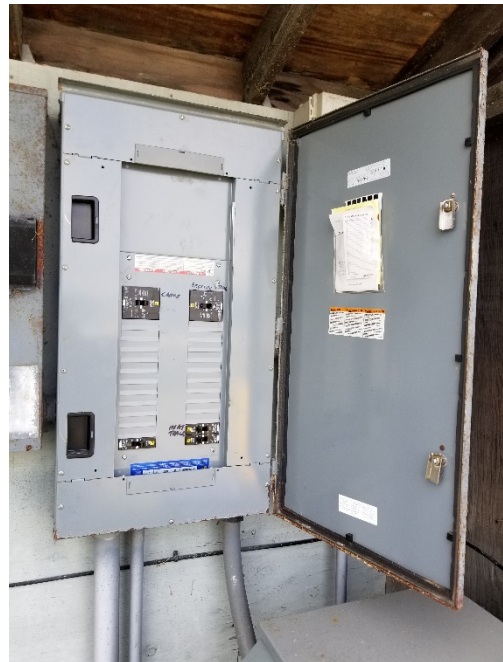
Photo 3: 480 Volt Distribution Panel
