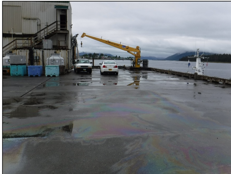
Typical ponding of water on main dock deck.
