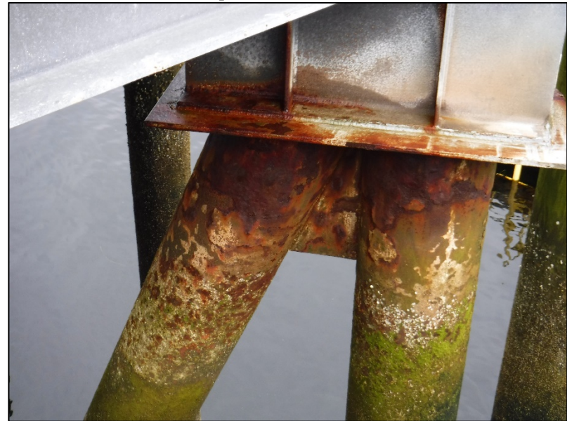
Typical corrosion of vertical/batter pile sub-cap weldment.
