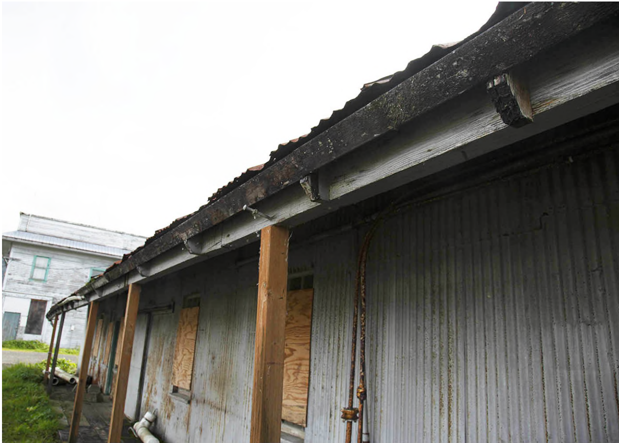
Figure 10. Maintenance Building, Wood Gutter. View Looking E.
