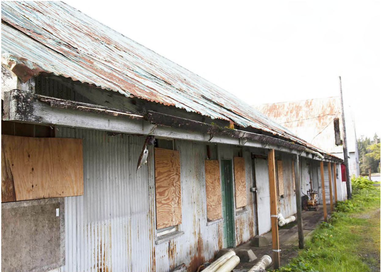
Figure 9. Maintenance Building, Wood Gutter. View Looking W.
