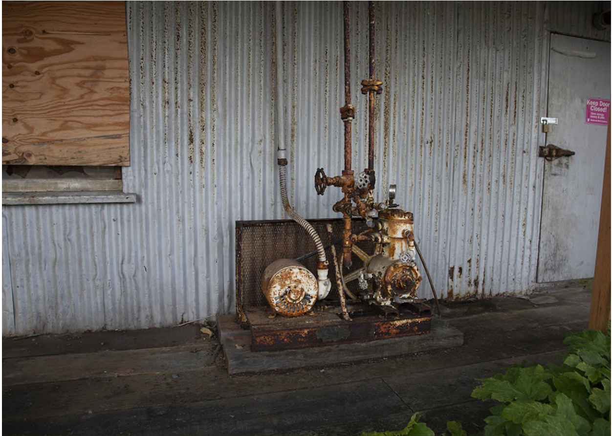
Figure 8. Maintenance Building, Cold Storage Compressor.
