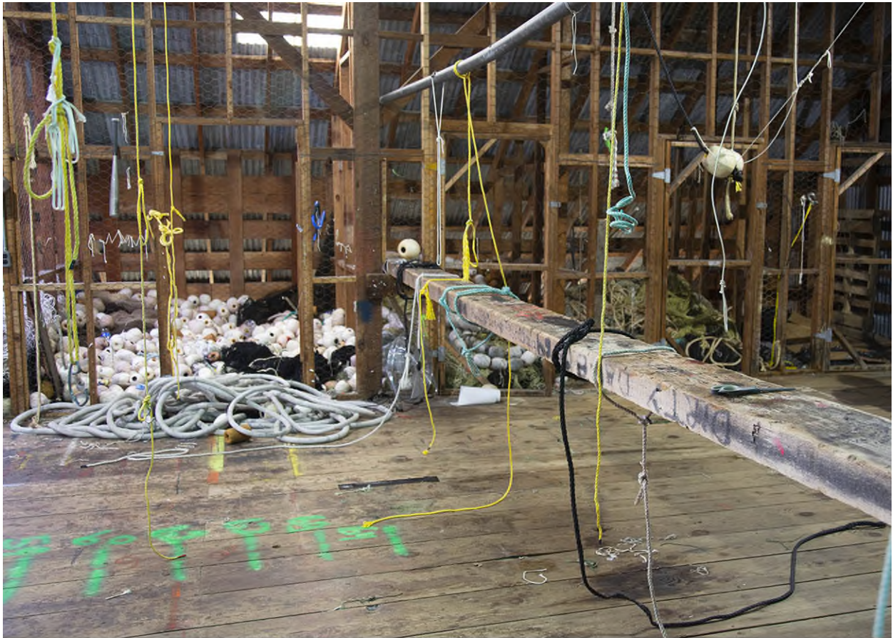
Figure 10. Web Loft, Interior Half Story (Loft), East Wall Gear Lockers. View Looking E.
