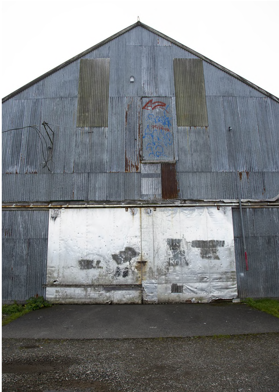
Figure 4. Web Loft, Service Doors and Second Story (Loft) Opening, North Facade. View Looking S.
