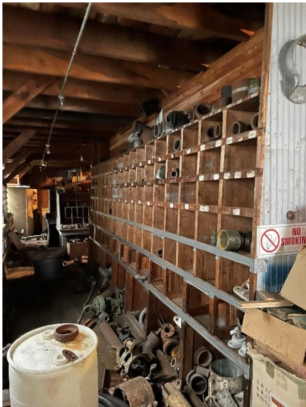
Typical open framing and storage bins
