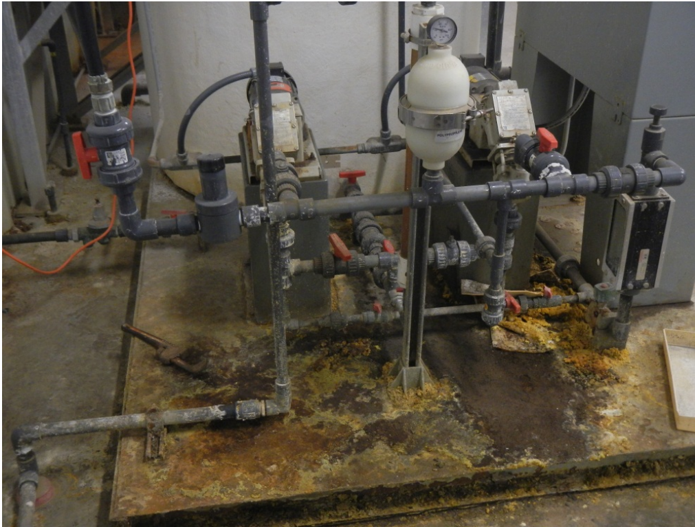
Figure 2.2: Corroded Alum Station
