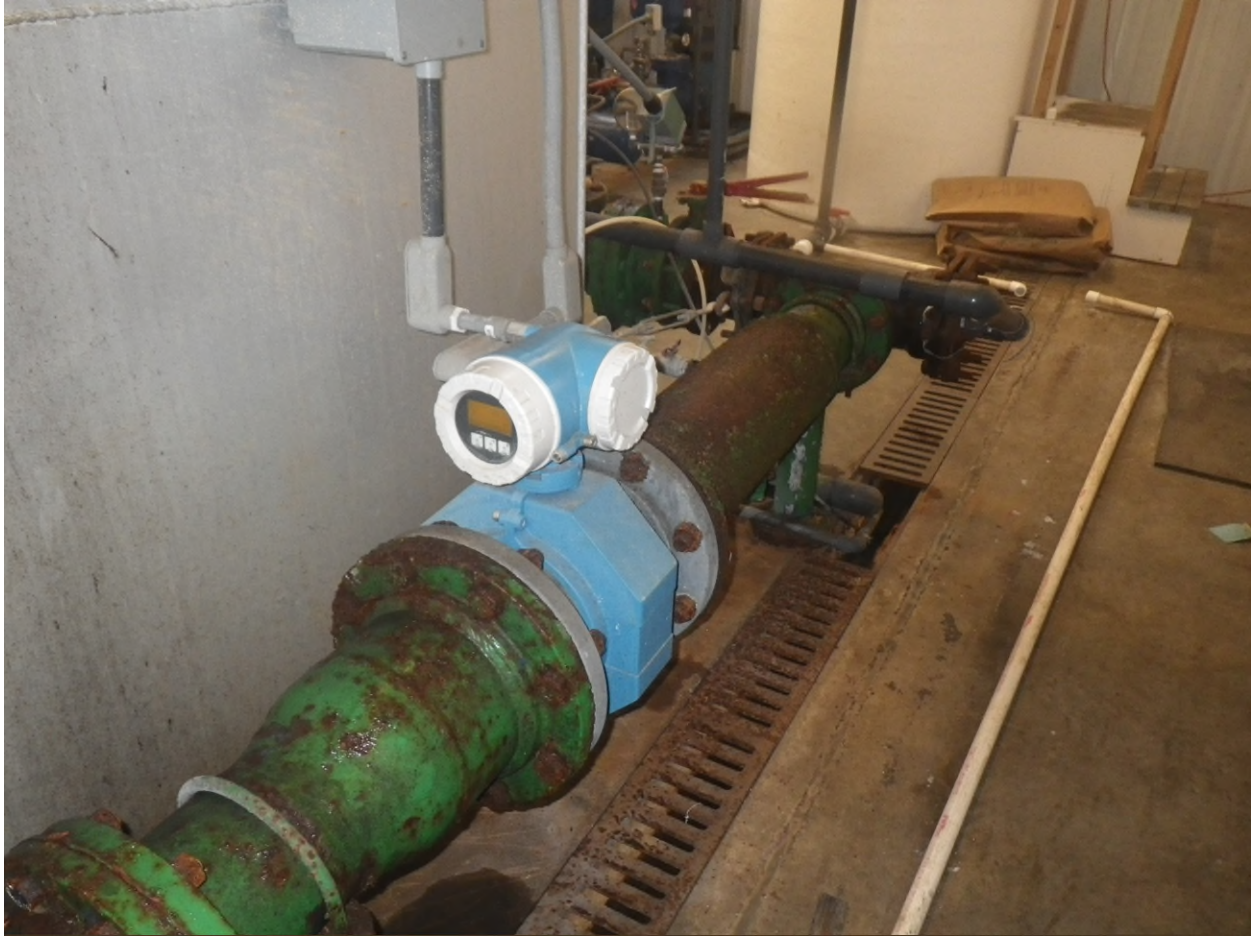
Figure 4 Master flow meter SCADA monitoring
