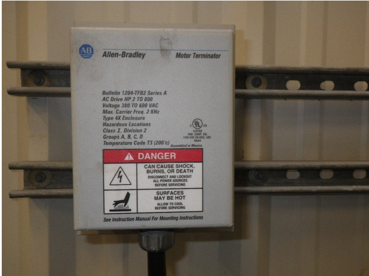
Figure 64 VFD/ Motor stuff
