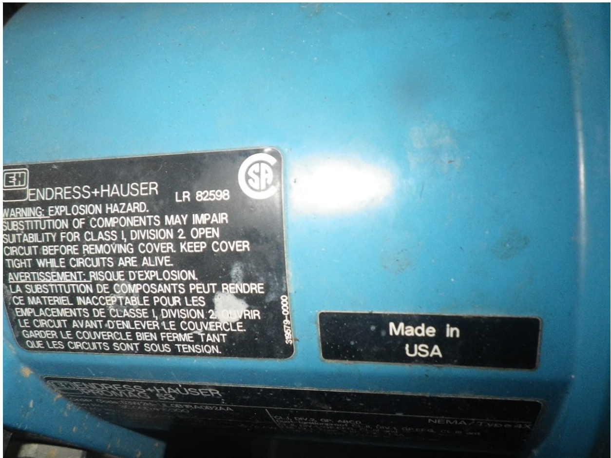
Figure 5 Master flow meter
