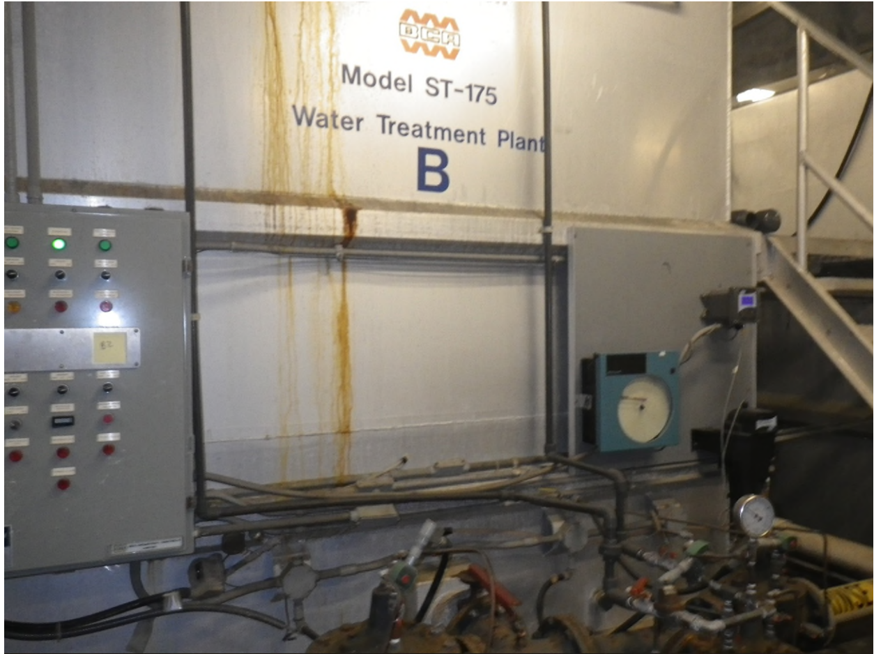
Figure 37 Filtration B2, chart recorder, and turbidity meter
