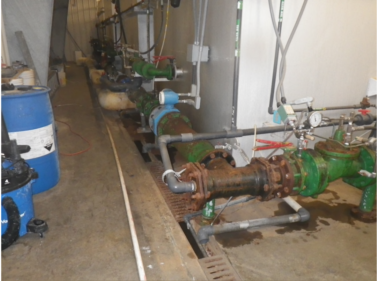
Figure 3 Chemical injection, Master flow meter, PLC controlled
