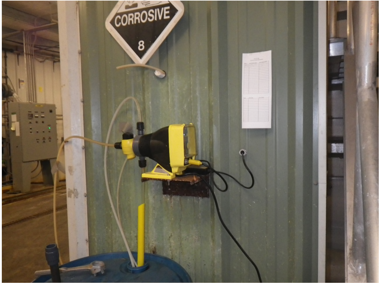
Figure 47 Chlorine Station, 4-20 MA
