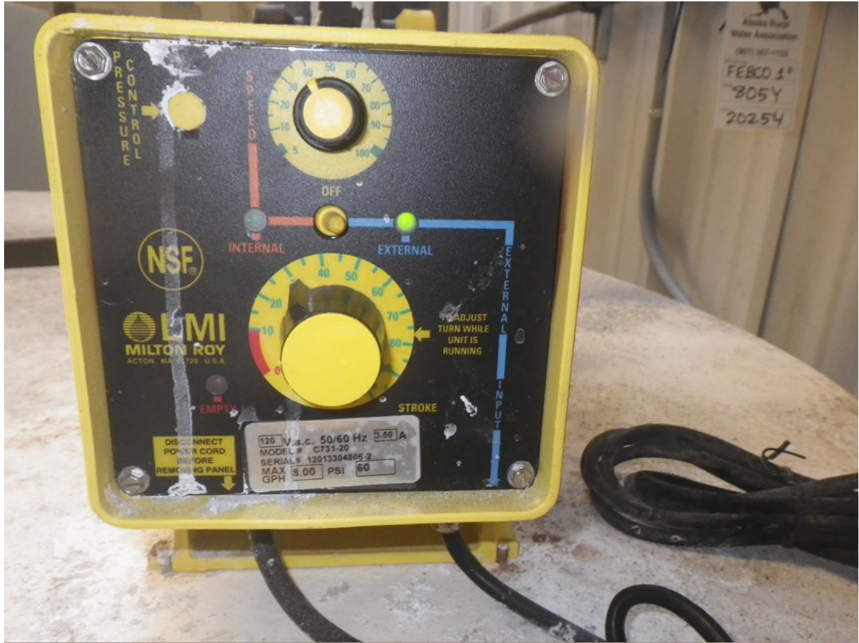
Figure 10 Soda Ash pump, 4-20 MA
