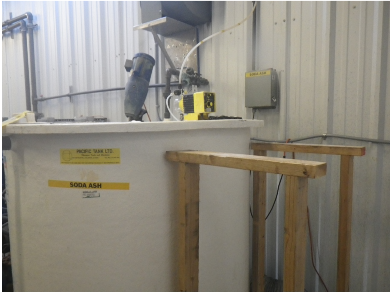
Figure 9 Soda Ash Slurry Station, 4-20 MA signal, PLC
