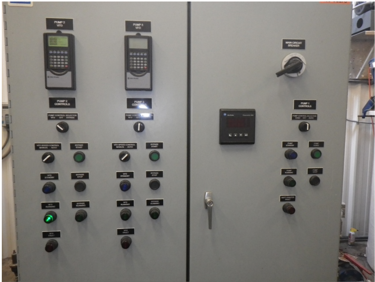
Figure 55 High Service pump panel
