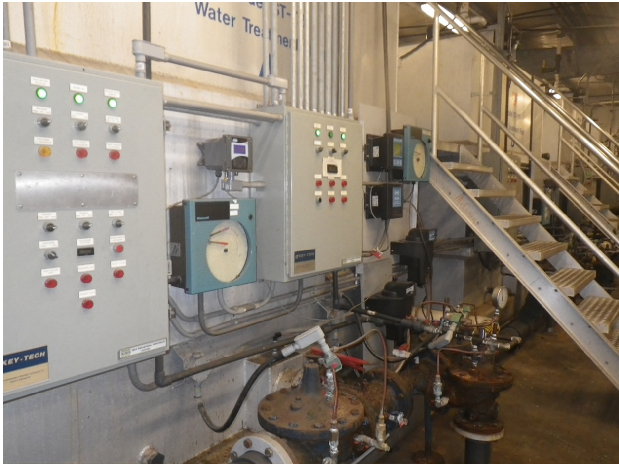
Figure 7 Filter 1A, chart recorder, master PLC
