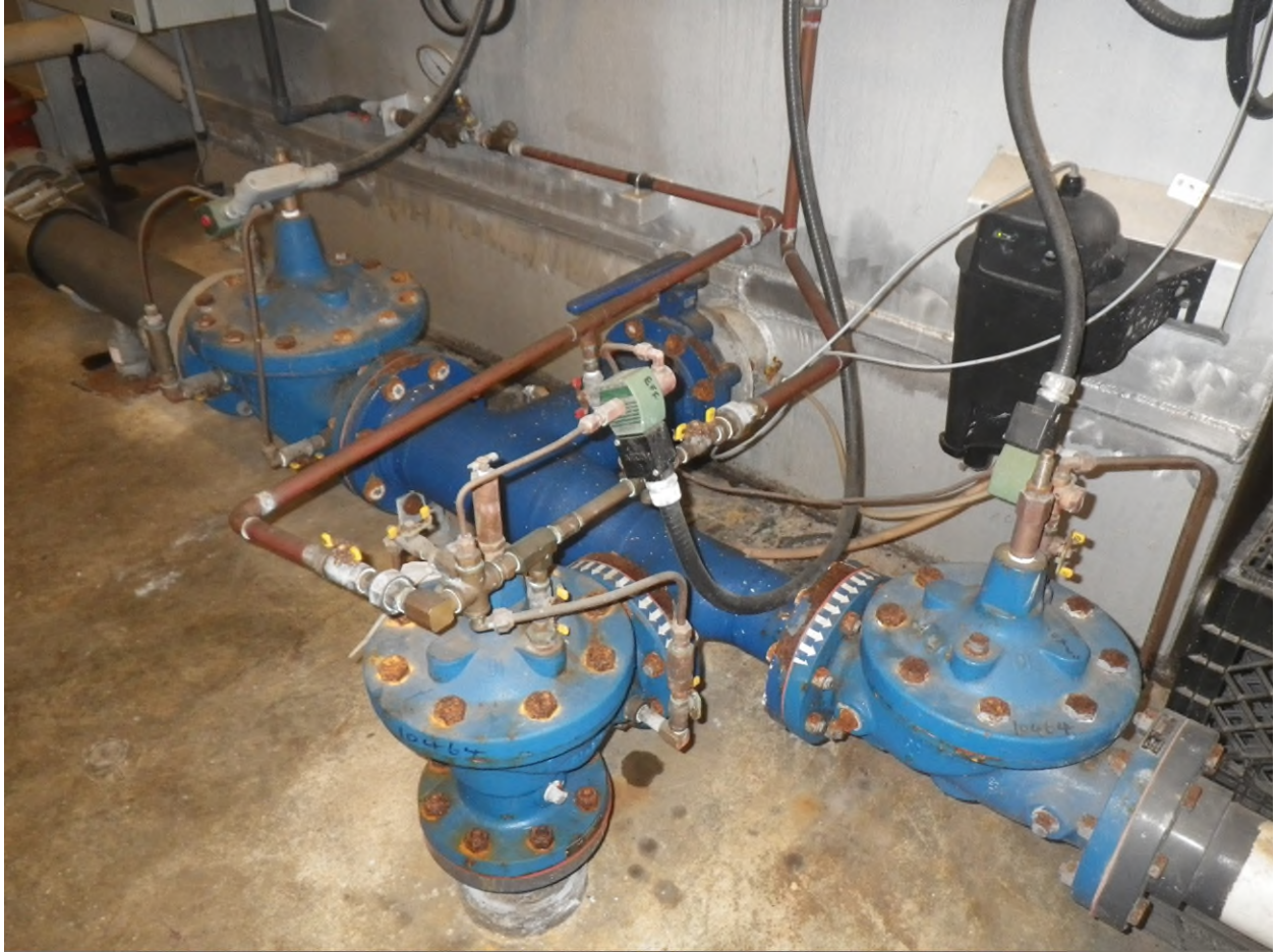
Figure 46 filter D4, plumbing
