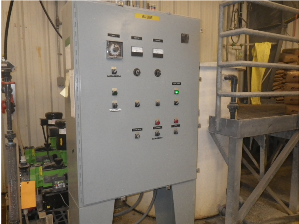
Figure 13 Alum Station, this is part of the original system, and the new system.
