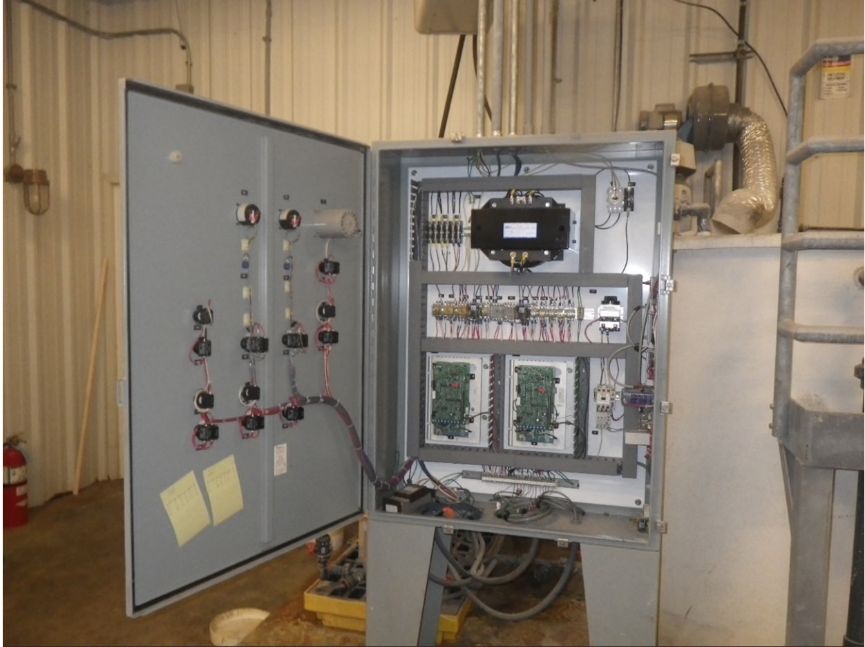
Figure 19 Alum Station, old pannel
